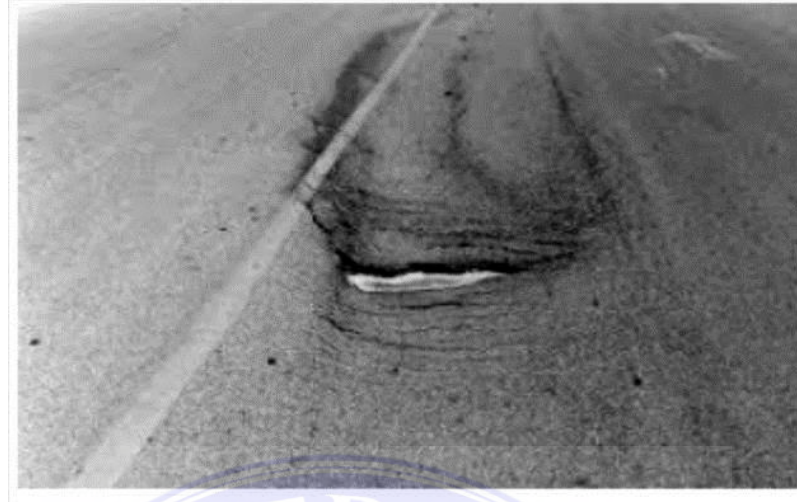
Gambar 33. Retak slip, (Shahin 2003)
