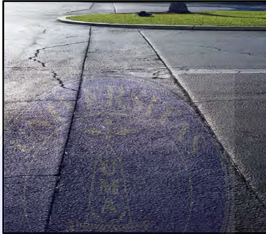
Gambar 22. Penurunan penanaman utilitas ( utility cut depression ) ( https://954asphalt.com/asphalt )
