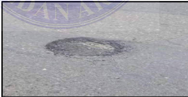
Gambar 17. Lubang ( pathholes ) ( https://dpu.kulonprogokab.go.id )
