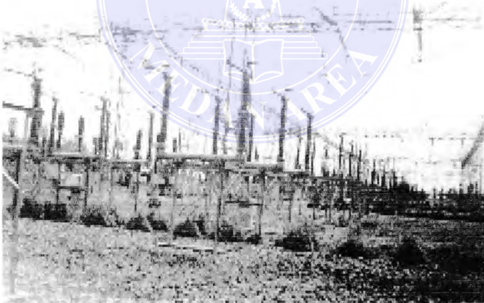
Gambar 3.6. Rel Daya ( Busbar)
