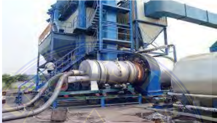
Gambar 2.5. Boiler jenis pulverizer
