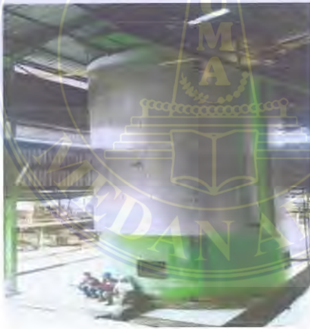
Gambar 3.14 Continous Settling Tank (CST)
