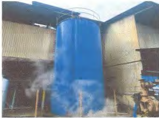
Gambar 3.21 Feed Water Tank
