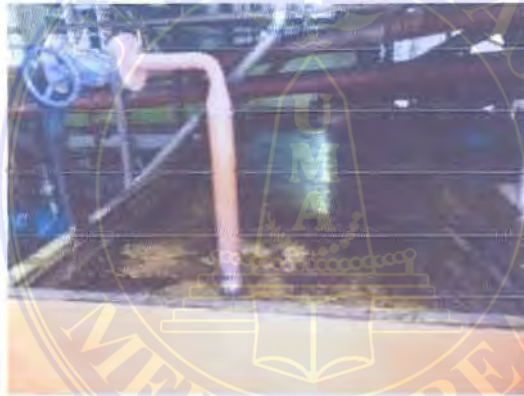
Gambar 3. 32 Sludge Drain Tank
