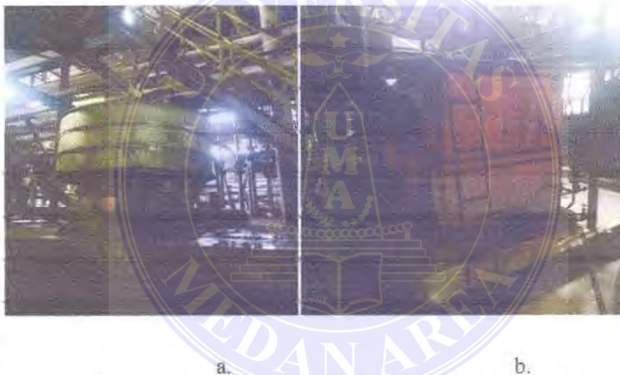
Gambar 3.11. (a) Oil Vibrating Screen (b) Crude Oil Tank
