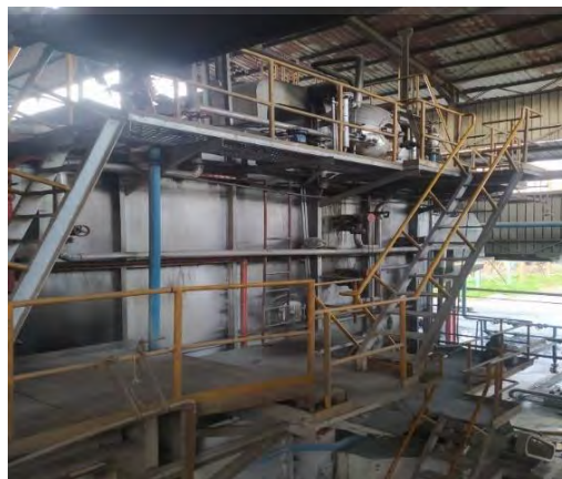
Gambar 3.3. Boiler PKS Pagar Merbau
