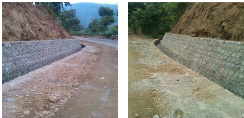
Figure 2.16 Drainage Construction Used For Water Drainage From Areas Owned By Roads That Are Often Damaged
