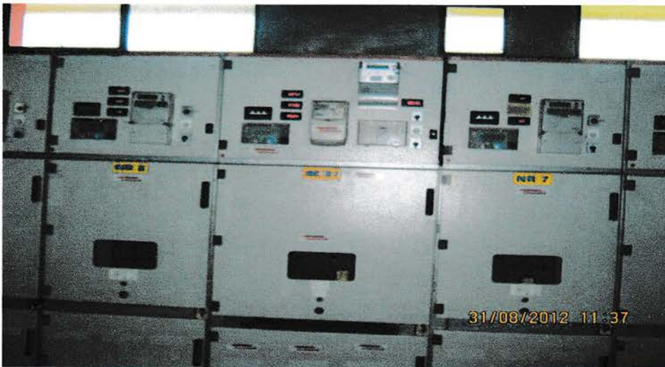
Gambar 2.19 : Panel Kontrol diruang control 20 KV
