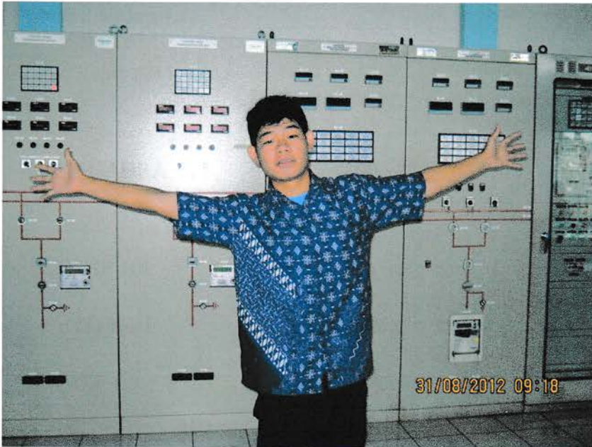
Gambar 2.18 : Panel Kontrol diruang control 150 KV
