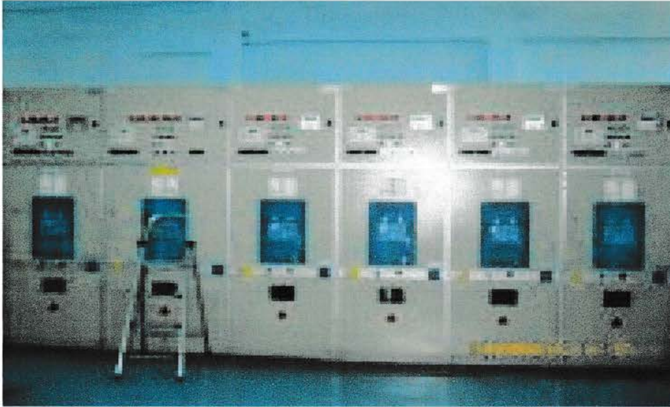
Gambar 2.20 : Panel Kontrol 20 KV
