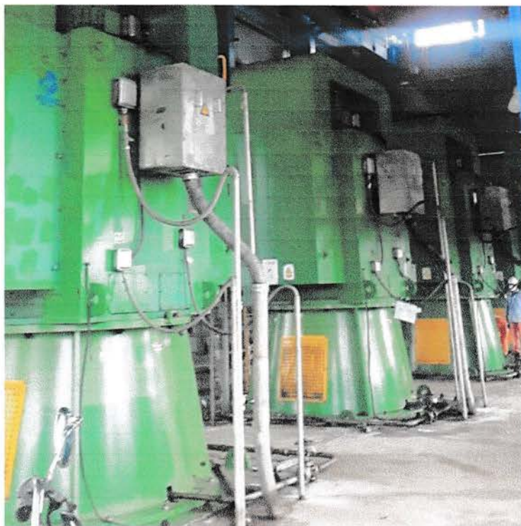
Gambar 3. 8. Circulating Water Pump PLTU Pangkalan Susu
