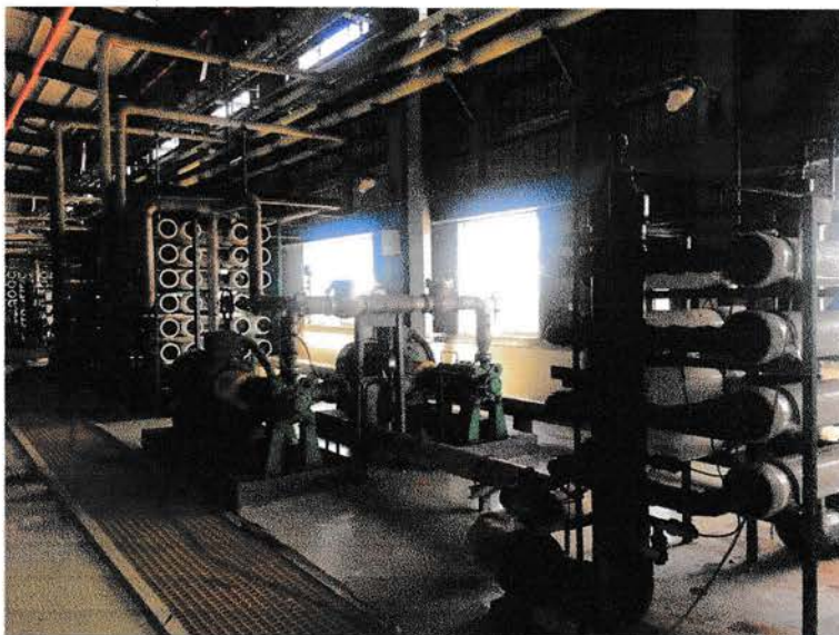
Gambar 3. 6. Fasilitas Reverse Osmosis PLTU Pangkalan Susu
