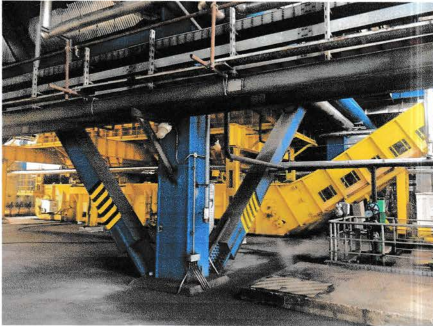
Gambar 3. 11. Submerge Scraper Conveyor PLTU Pangkalan Susu
