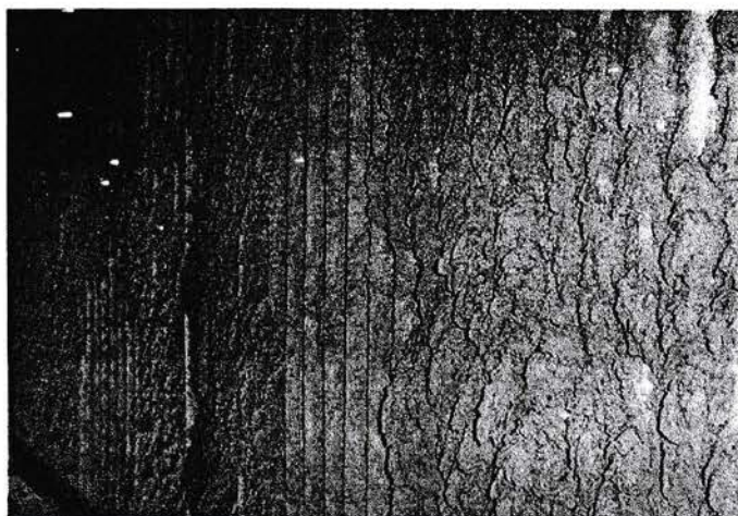
Gambar 3. 18. Wall Tube Boiler
