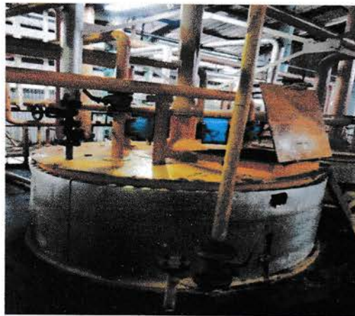
Gambar 3.14 Tangki Clean Oil Tank
