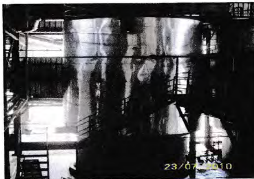
Gambar 3.7 Continuous Settling Tank
