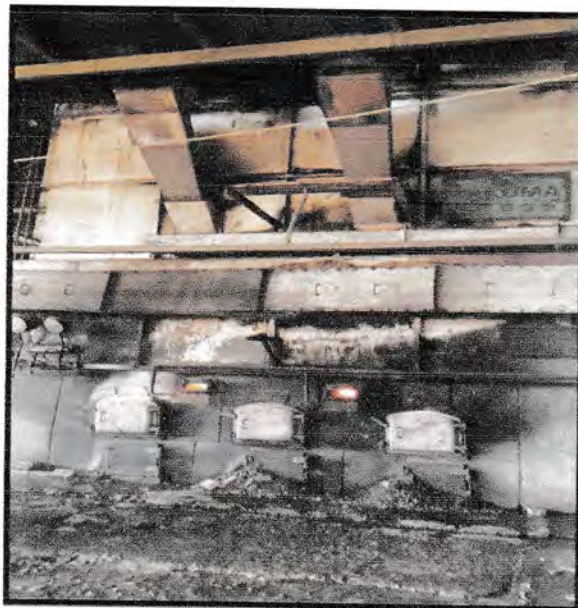
Gambar 3.25 Boiler Merk Takuma
