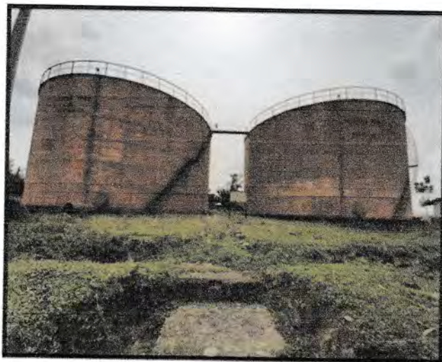
Gambar 3.24 Storage Tank 2000 Ton
