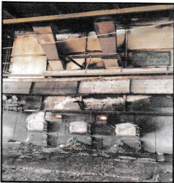
Gambar 3.25 Boiler Merk Takuma
