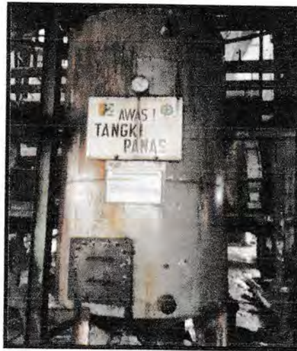
Gambar 3.19 Sand trap tank
