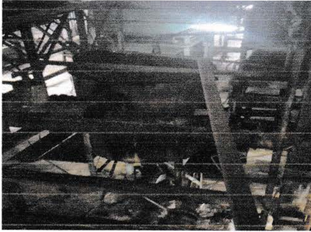
Gambar 5.9. Sand Trap Tank
