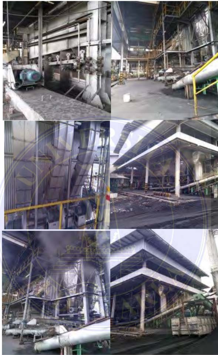
Figure 3.2 boiler at PT. Valley Bhakti Plantation, Agro Lestari Aceh Singkil.
